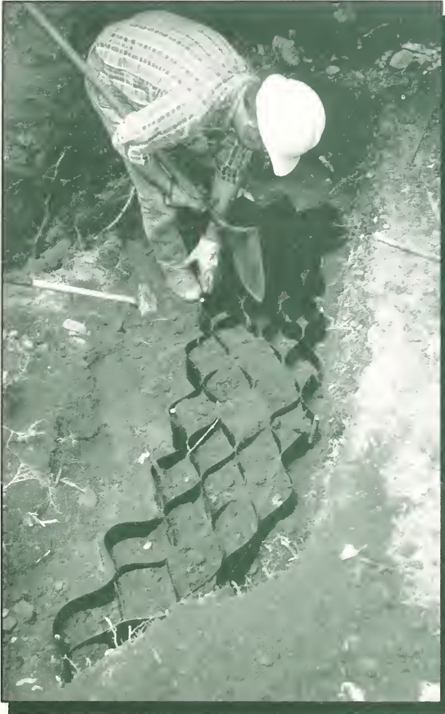
Figure 72—Geocell usually has geotextile underneath to provide separation from saturated soils. Here a narrow strip of geocell is the first course of a retaining wall.
